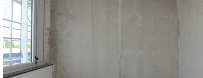
Untreated concrete surface
