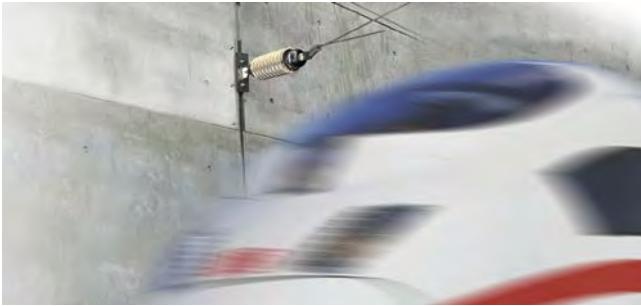
Overhead lines in tunnels
