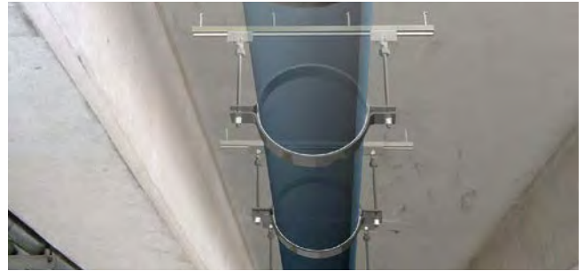
Pipe suspension under bridges
