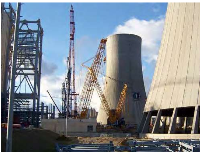
Neurath power plant in Grevenbroich, Germany
