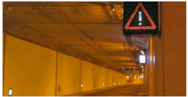
Lighting and signalling systems
